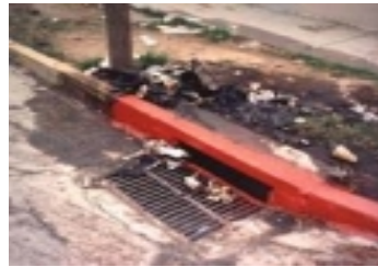
Dirty Storm Drain
